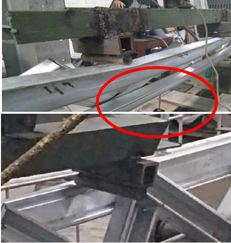
Picture 7. Failure of B-I Non Centric C Profile Beam
