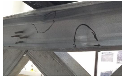
Picture 9. Failure of B-III Non Centric C Profile Beam
