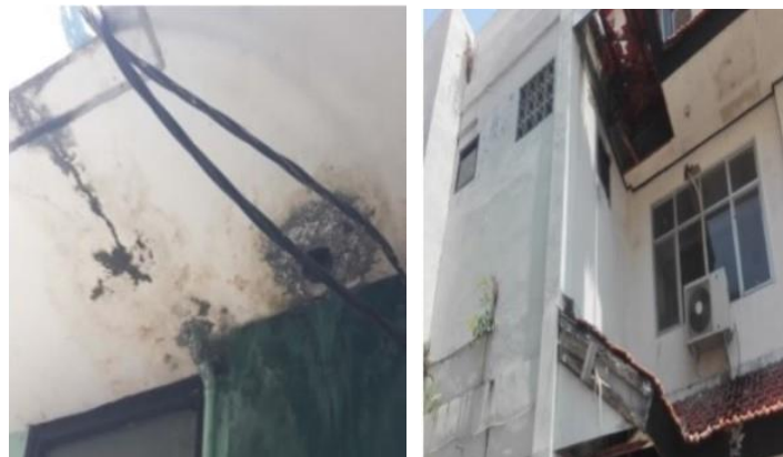
Picture 3. Moderate level of damage
